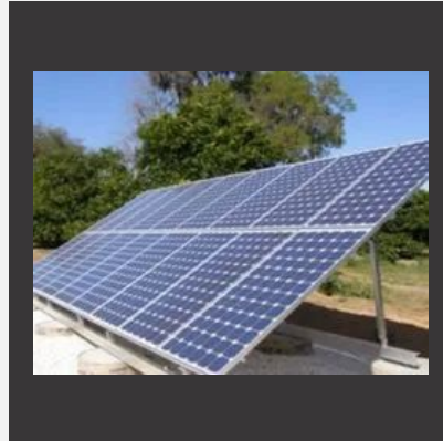
Solar Renewable Energy Systems
