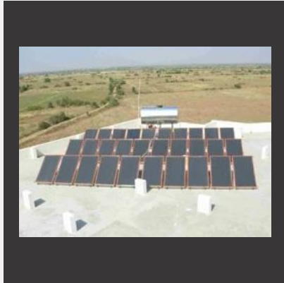
Industrial Solar Water Heater
